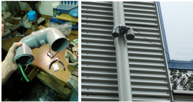
The fine dust sensor mounted to our school building.
